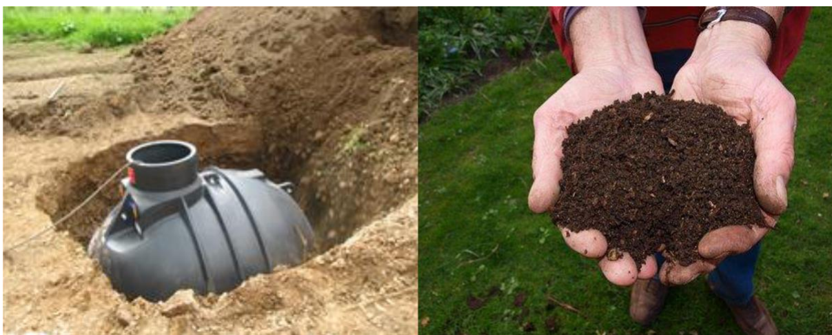
Figure 35:(left) sludge storage tank (photo: U.Strniša); (right) compost (photo: pixabay)
